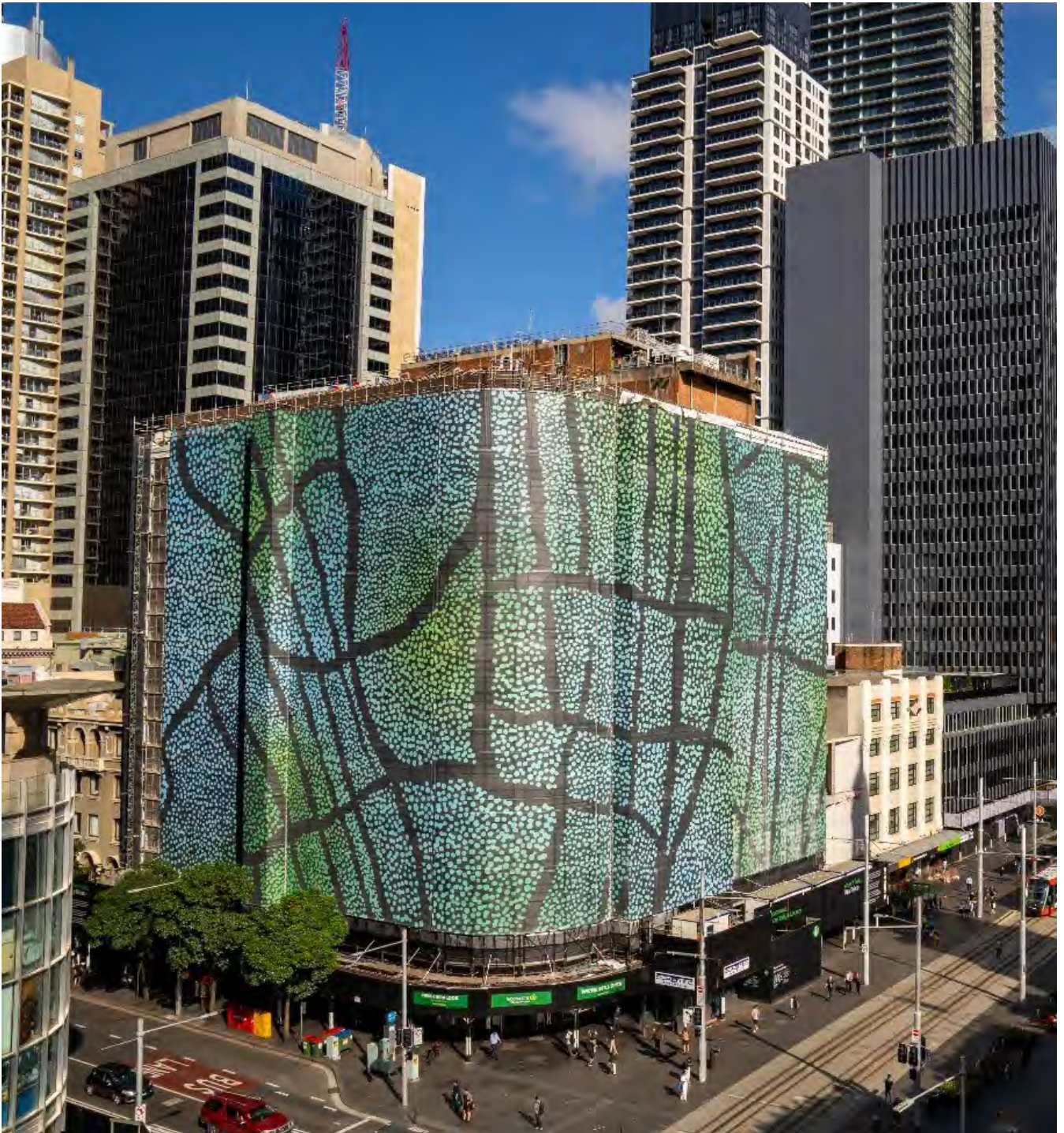
Figure 11. Creative hoardings covering the Woolworths Building during its renovation, April 2022 - Photo by Abril Felman/ City of Sydney
